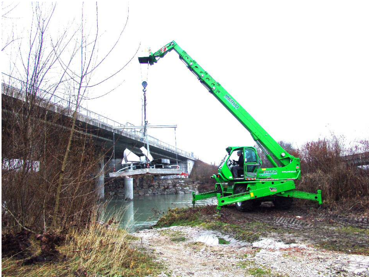
Picture from October 2009 th year: Smaller unit SP 1 on a concrete basement plate, during assembly on the bottom of a slow river stream near Ljubljana.
